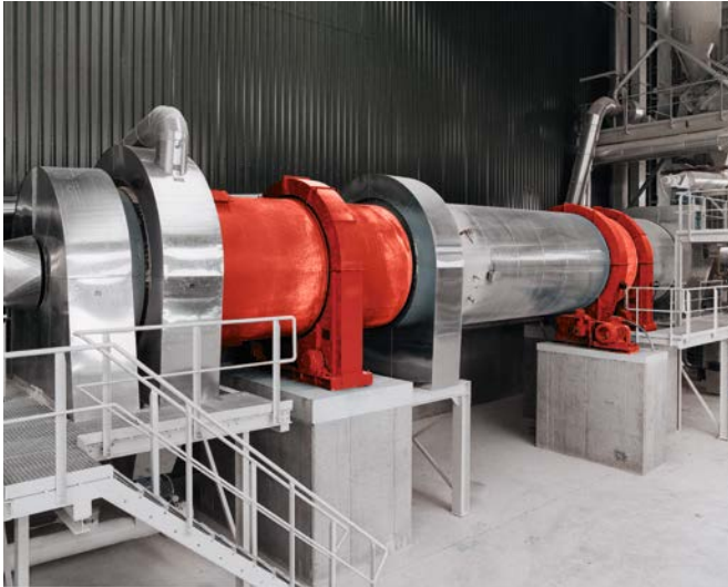
Rotary tubular calciner with integrated cooler
