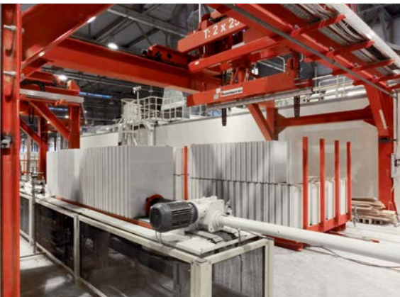
Gypsum block unloading and compacting unit
