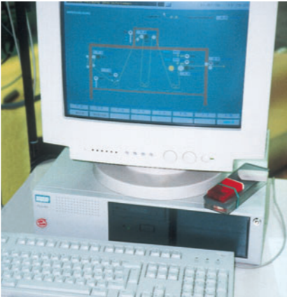
System control using a programmable controller and visualisation system
